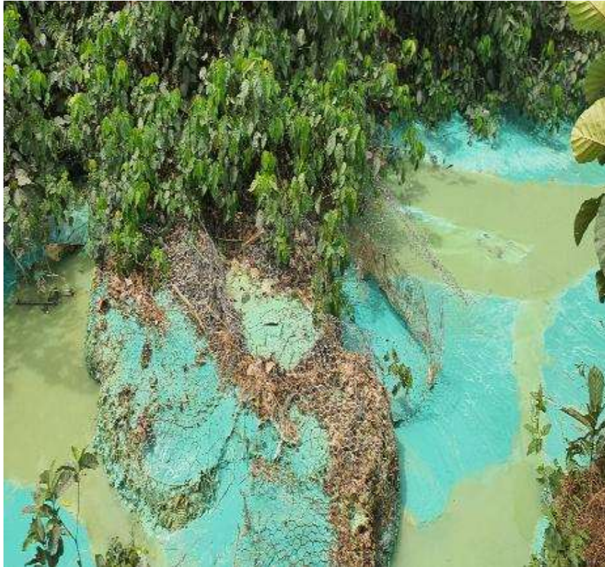
Damaged Gabion Basket observed at the TSF-R
